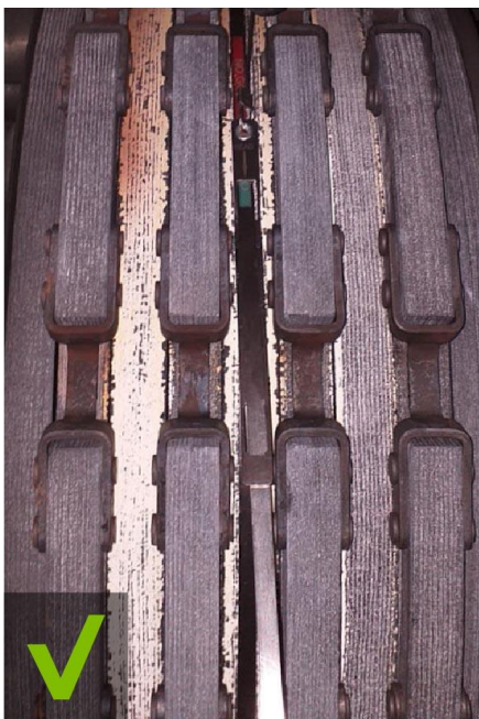
No sign of oxidation
