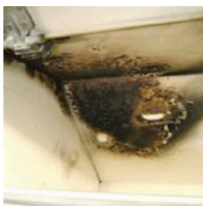
Damage to cabin overhead compartment video camera
