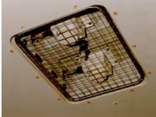
Smoke detectors and Extinguishing nozzle
