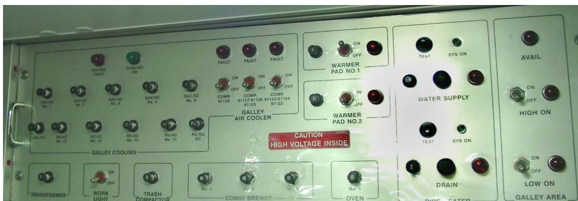
Example of Galley Circuit Breaker Panel
