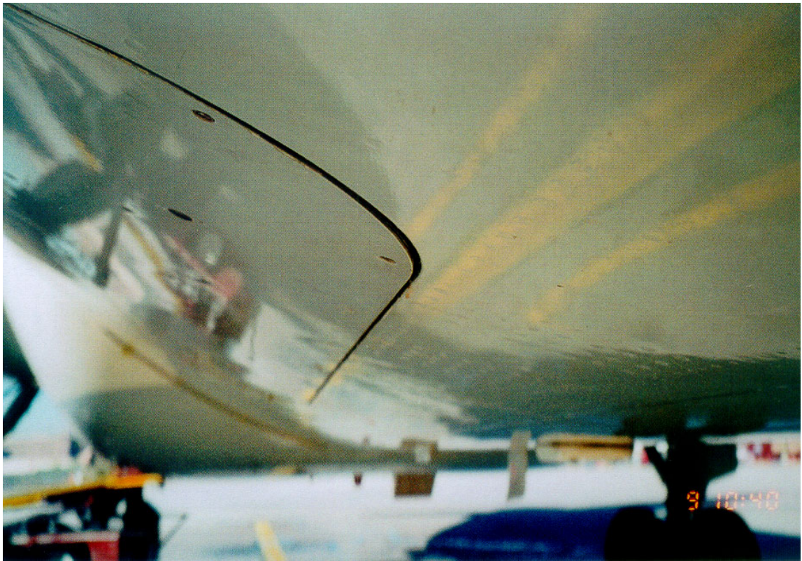
Mismatched access doors
